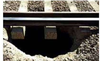
Sinkhole under railway tracks
